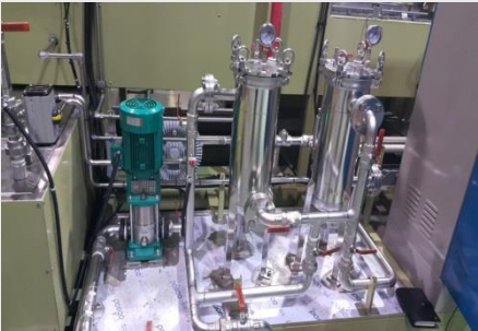
Line-feed pump & filter
