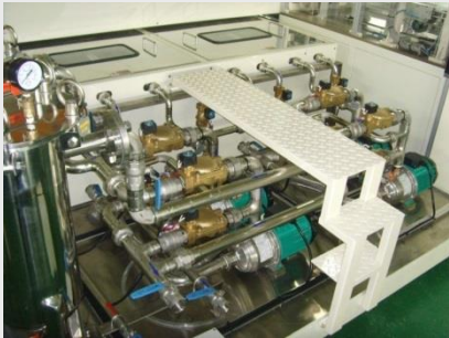
Tank &amp; Pump-line
